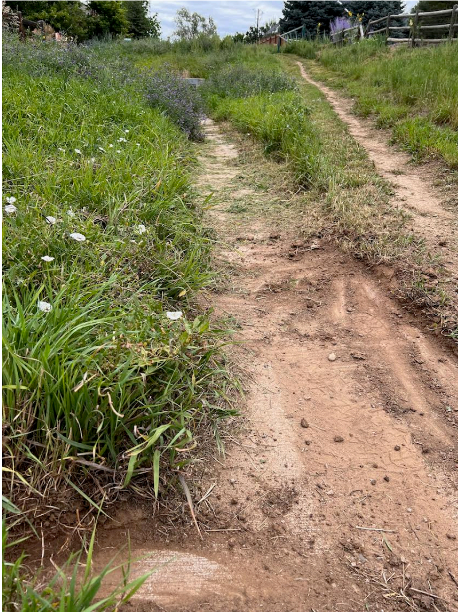
Left edge covering 12"+ of drainage concrete
