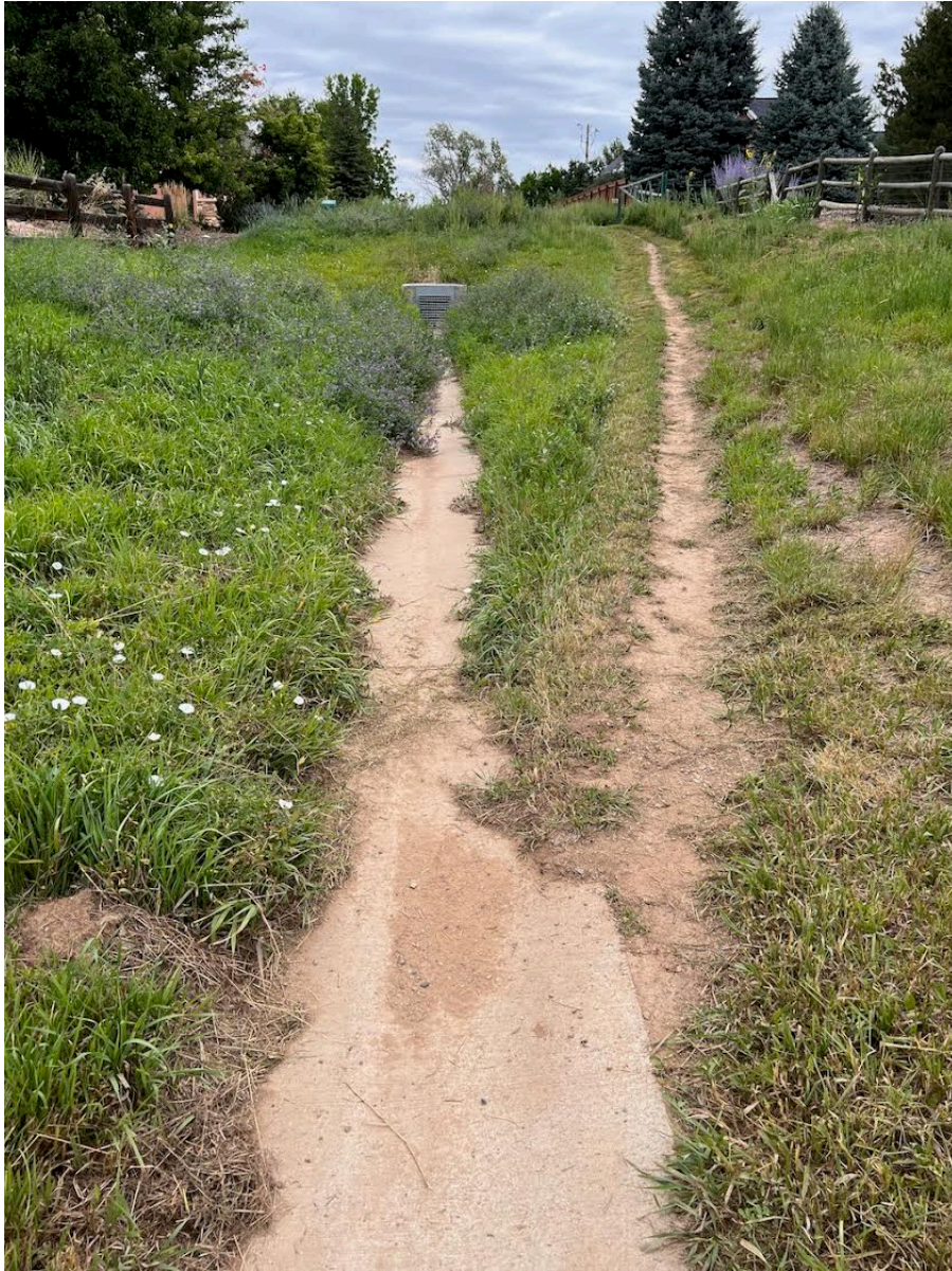
Note Mr. Denenberg is mowing up this dirt path to the right (both sides), but not mowing the remaining channel for about 50 feet going into the culvert.
