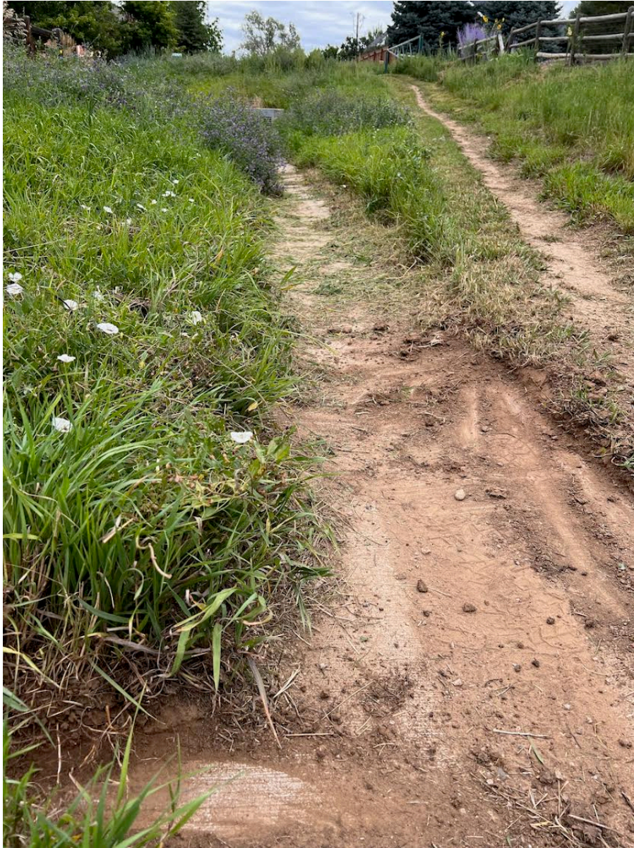
Left edge covering 12"+ of drainage concrete
