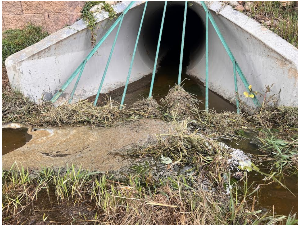
Algae formations on the water indicating long-term blockage
