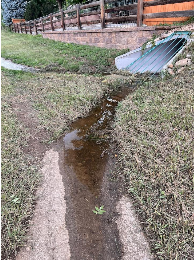
Stagnant pool forming at South End culvert
